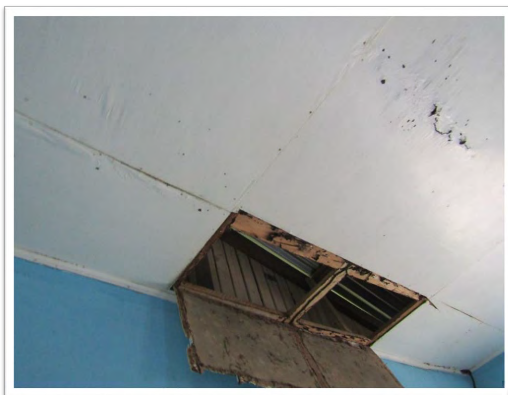
Figure 10 - Picture showing dilapidated ceiling at Agatash Primary School Source: Audit Office of Guyana
